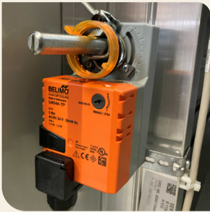
Figure 3. Actuator for outside air damper
