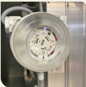
Figure 5. External pressure differential sensor across the air intake filter
